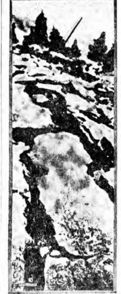
This was a stretch of the excellent motor highway between Tokyo and Yokohama. Then came the earthquake, and the solid ground was broken into gaping chasms often many feet deep. In Yokohama and else where the surface of the ground suddenly sank at least three feet; the faces of mountains were split with great cracks; islands, like the beautiful Oshima, sank below the surface of the water, and other islands were thrust upward from the depths.
